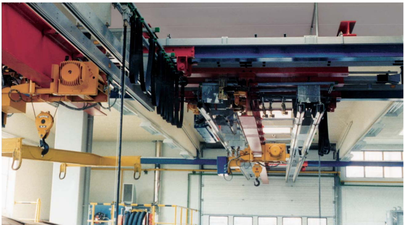
Aluminium enclosed conductor system on crane bridge.
