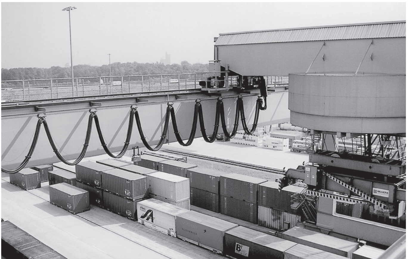
Cable carrier at a container crane
